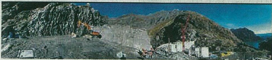
Vieux Emosson Dam, the most spectacular hydropower construction sites in Swiss Alps in Switzerland.
